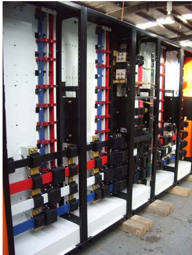
Rear of switchboard showing busbars insulated by rigid sleeving and busbar joint covers. (Picture by kind permission, SRS COMCELL SWITCHBOARDS)
